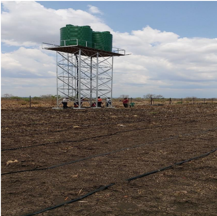
Figure 1: Water tanks installed at Katapazi Irrigation Scheme in Zambia
