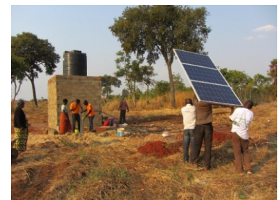
Installation of Solar Panels for irrigation purpose at SOS School in Chipata, Eastern Zambia.
